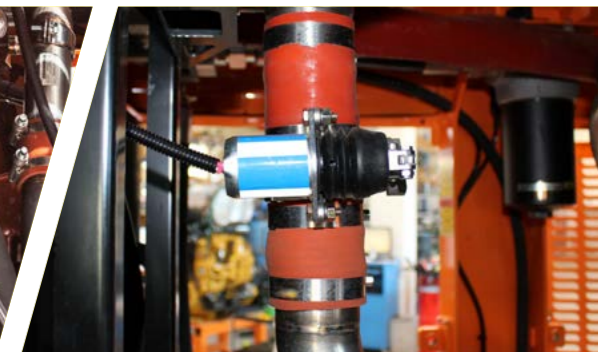
Air shutoff valve
