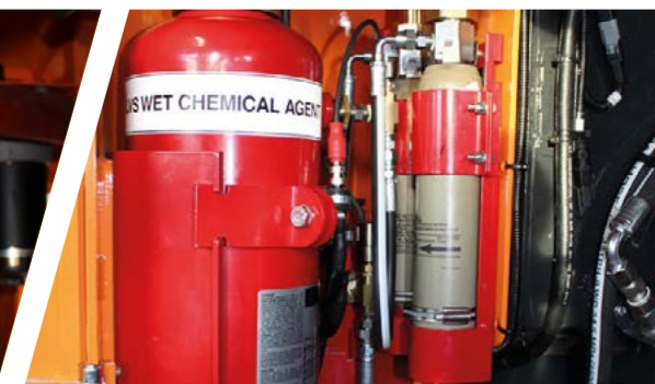
Automatic fire-extinguishing system
